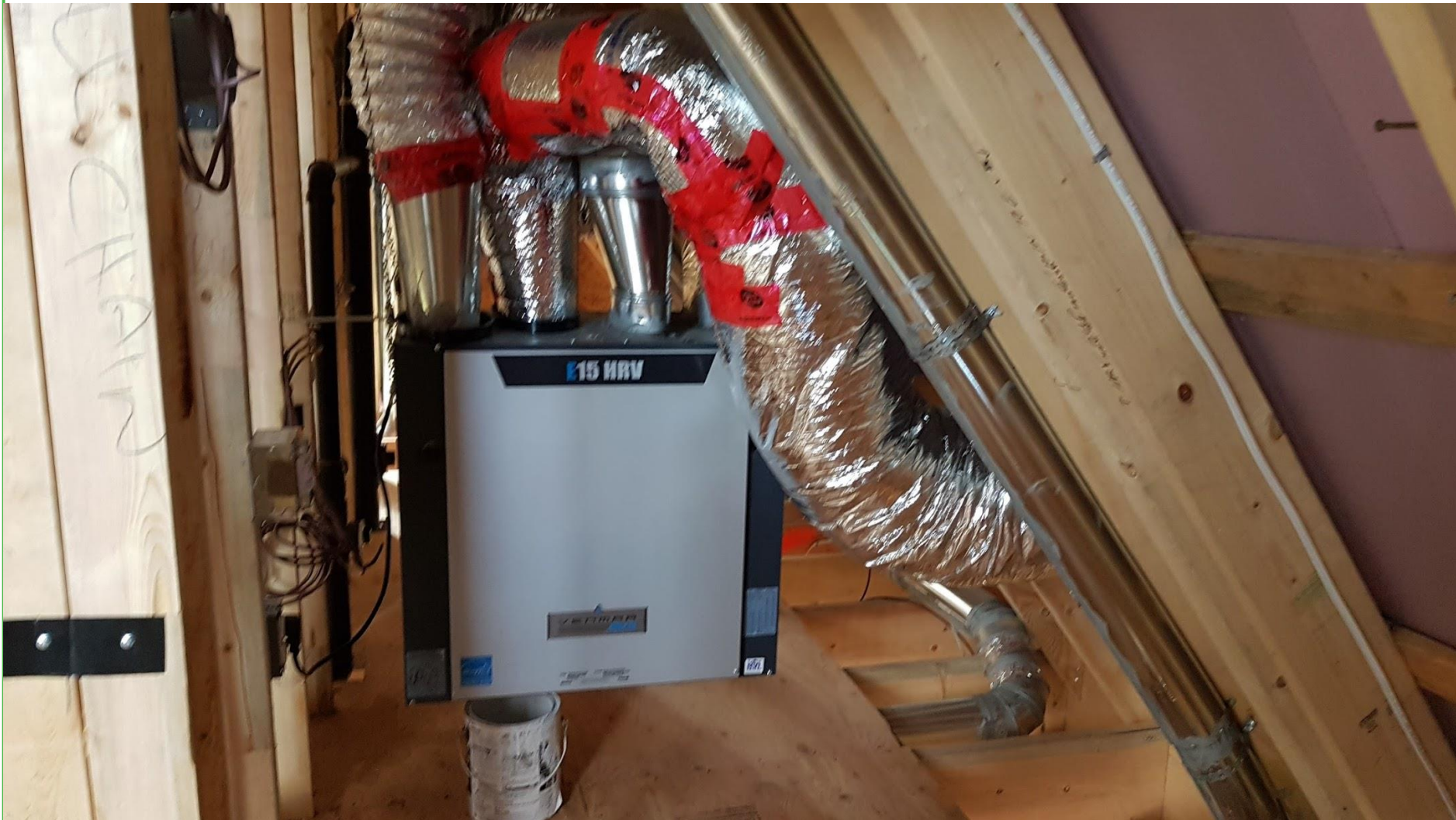
Installed HRV in conditioned (warm) attic space.
