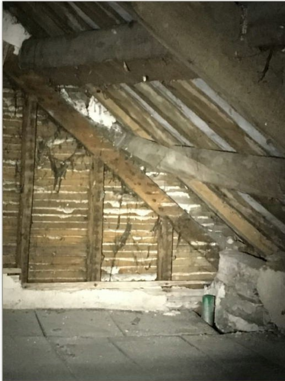
Picture 10 Split purling at the loft space, the roof is lacking vertical support. The rafters will spread outwards. Most of the timbers seem having gained moisture which seems to have halved their strength.
