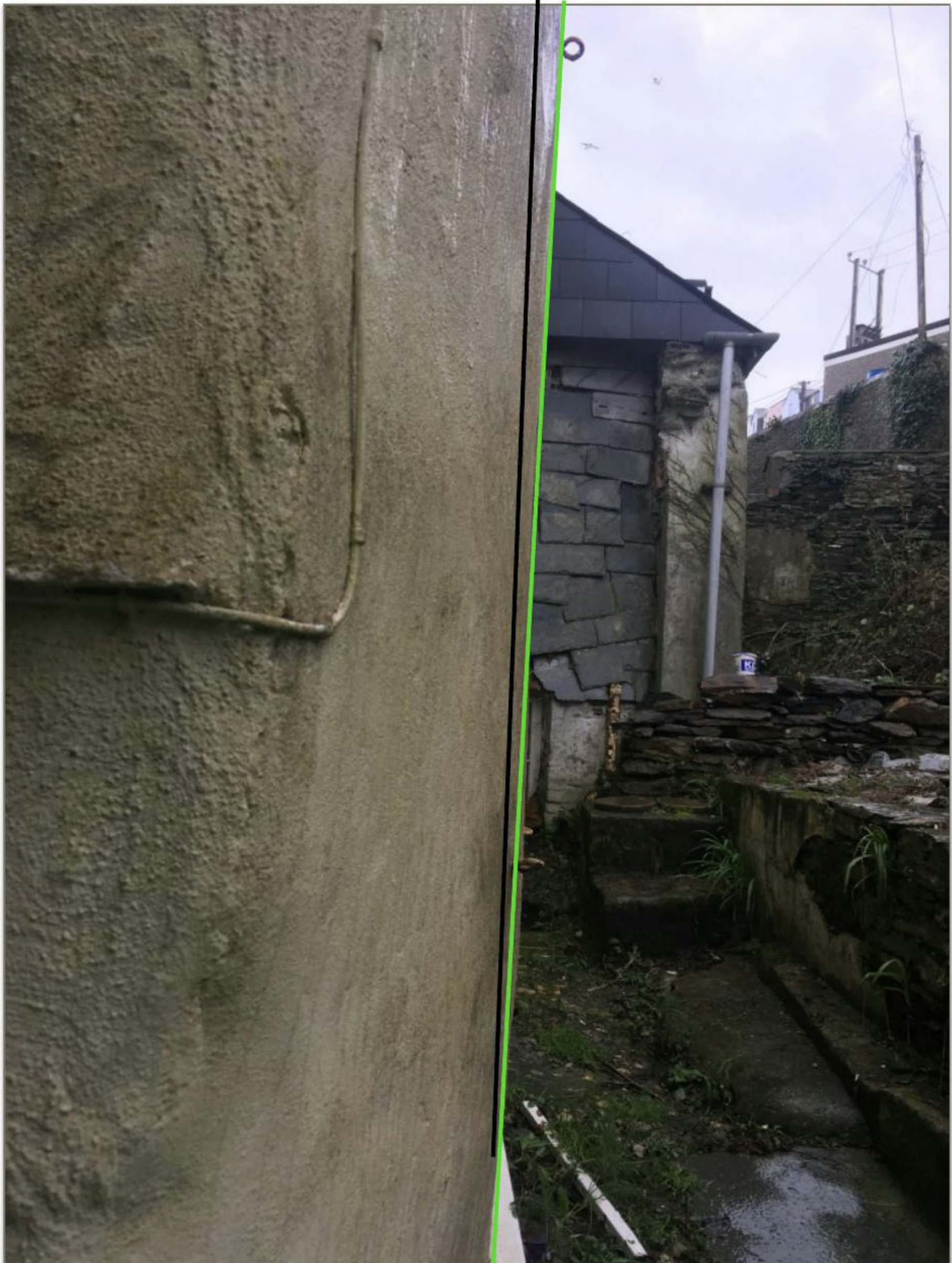
Picture 7 The rear elevation is leaning approximately 12 degrees (Note the black line is not vertical)
