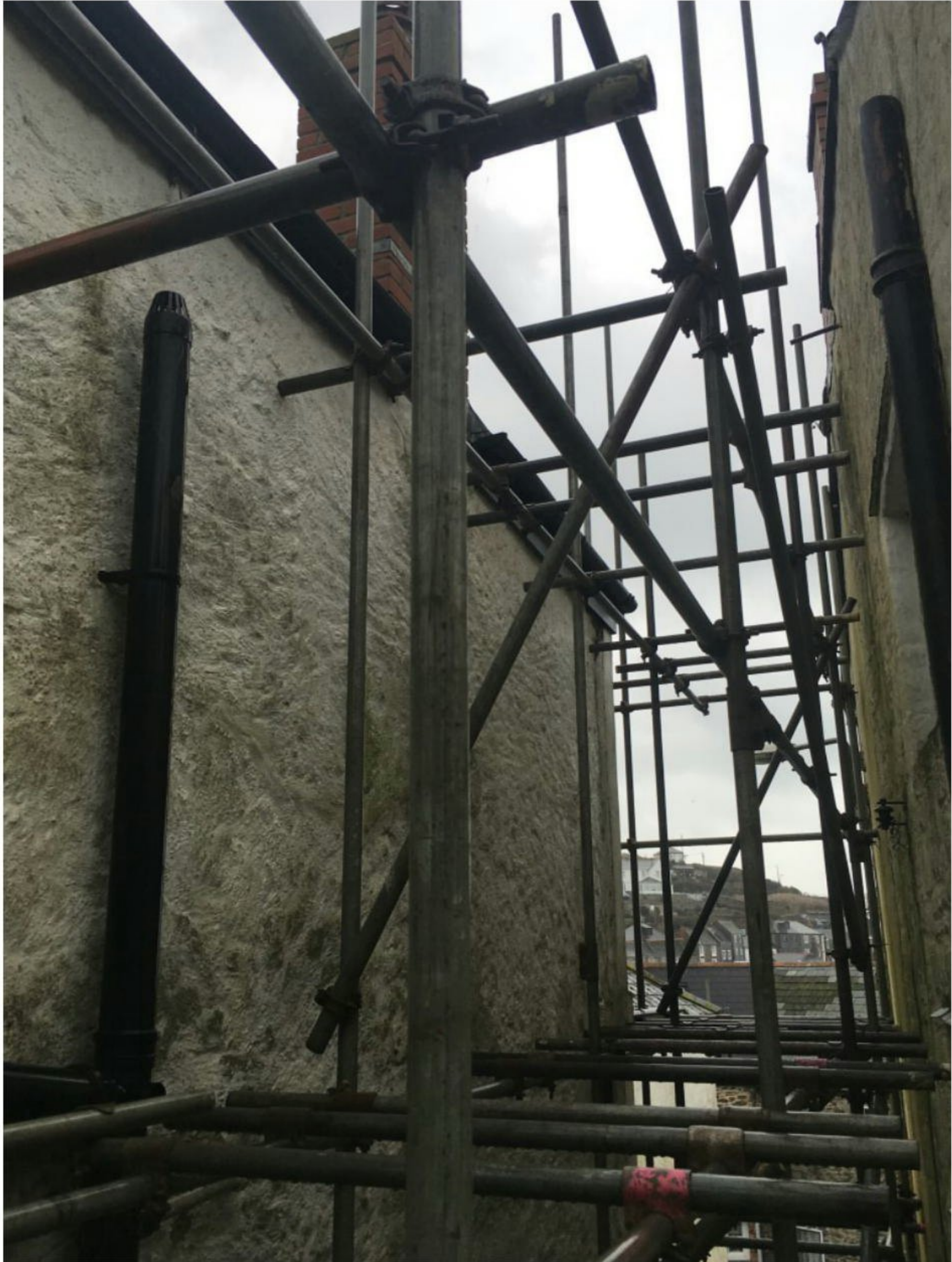
Picture 14 Scaffolding at the side elevation. Note the chimney stack was only renovated at the top.
