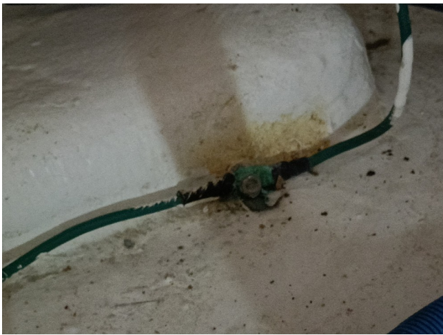
Figura 8: ground wire with few oxid- left stern
