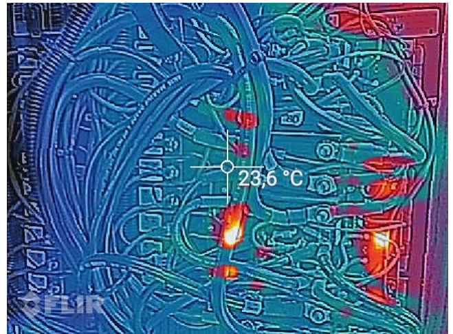
Figura 7: thermal camera inspection for electric panel
