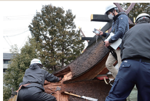
An on-the-ground survey of fire damage on the cypress-bark roof of Sudōtennō-sha Shrine (Nara City, Nara Prefecture) (Cultural Heritage Disaster Risk Management Center)
