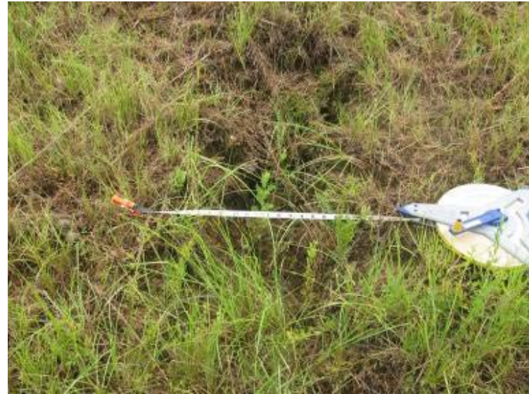
Photo 134: Rill located on north exterior slope of Process Sedimentation Pond (typical of six).
