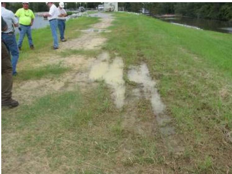
Photo 57: Ruts and ponding of water on crest southwest embankment of Ash Pond.
