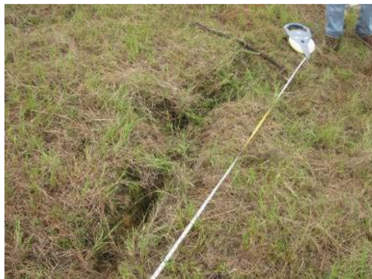
Photo 132: Approximate 16-foot long rill erosion on north exterior slope of Process Sedimentation Pond (Depth x Width ~1 foot, respectively).
