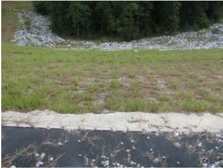
Photo 149: Emergency spillway/ articulated concrete block mattress located on east exterior slope of Process Sedimentation Pond looking east (down slope).
