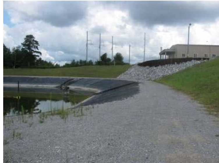
Photo 178: South crest and interior slope of Process Return Water Pond looking east. Note presence of textured HDPE liner on interior slope (typical).
