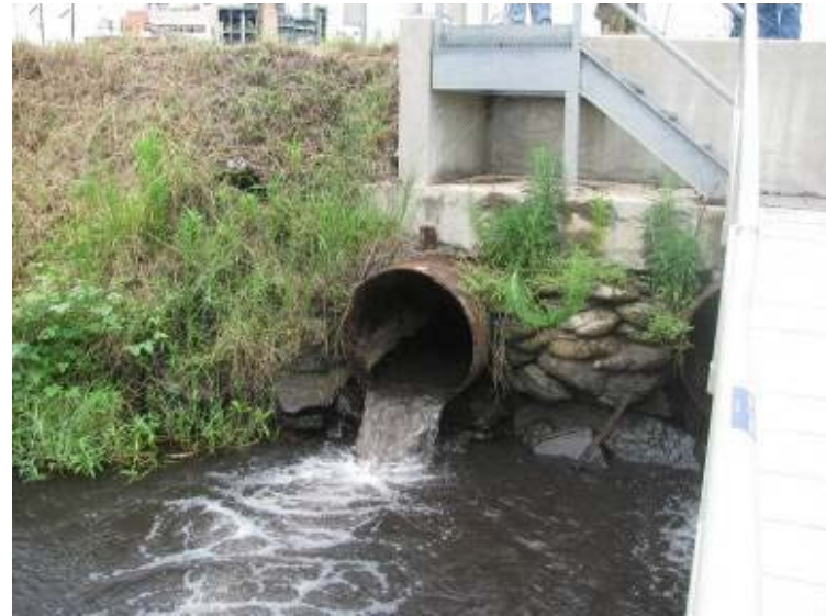
Photo 78: 30-inch diameter inlet pipes at north corner of Ash pond looking northwest.
