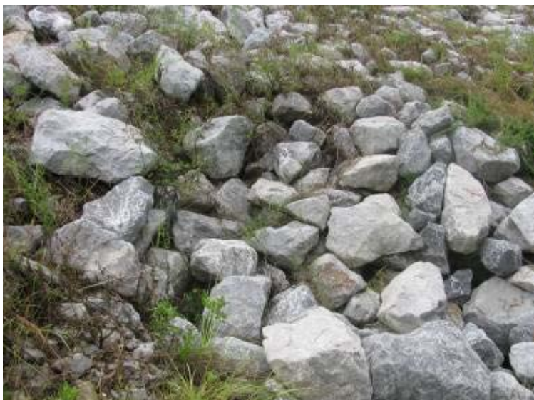
Photo 125: Riprap slope protection along toe of west exterior slope of Gypsum O Pond looking east. Note exposed filter fabric.
