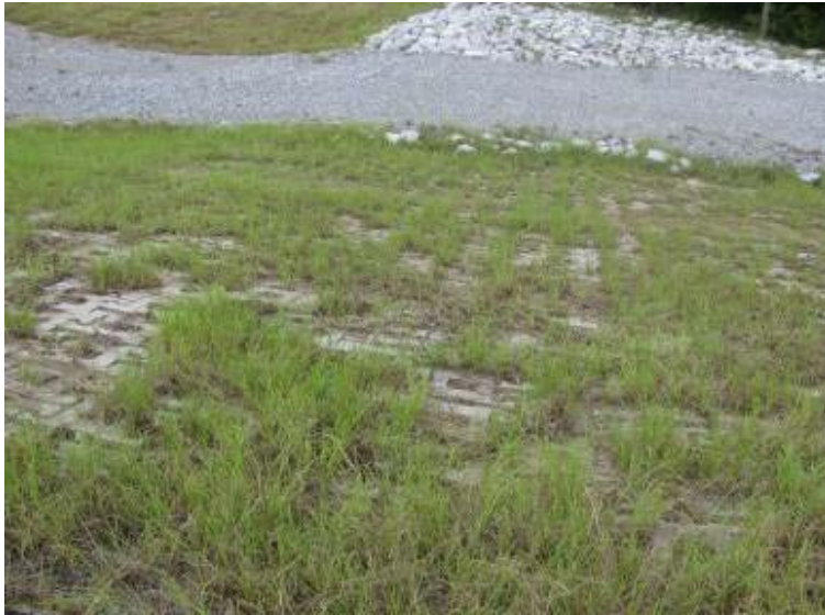
Photo 189: Emergency spillway/ACBM located on west exterior slope of Process Return Water Pond looking west (down slope).
