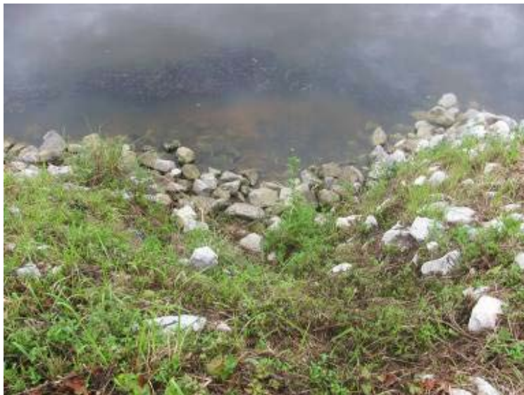
Photo 15: View of rill at exterior toe of slope of Ash Pond along Northeast embankment looking east.
