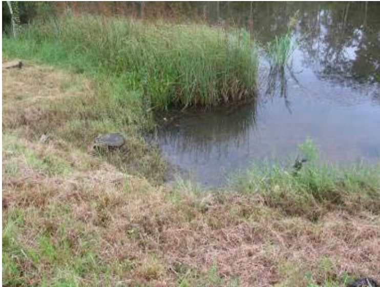
Photo 29: Scarp at toe of slope of Ash Pond along southwest corner.
