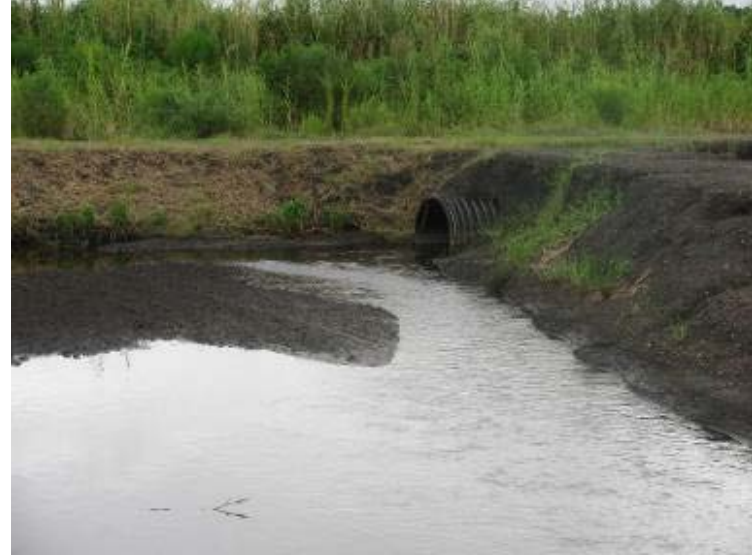
Photo 90: Interior slopes, divider and surface of Decant/Settling Pond #2 looking southeast. Note presence of ash/CCW.
