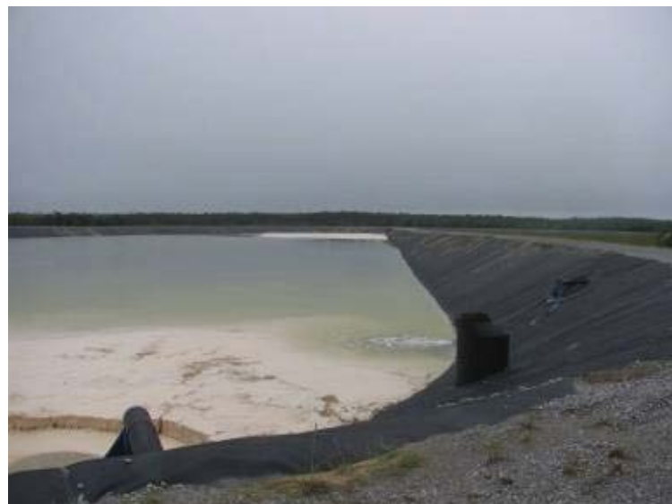
Photo 102: View of surface and south interior slope of Gypsum Pond looking northwest. Note discharge pipe and deposition of gypsum in foreground.
