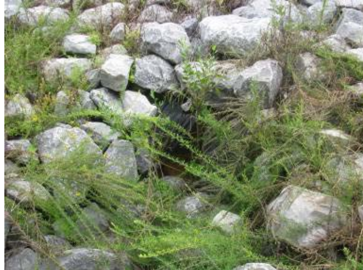
Photo 124: Riprap slope protection along toe of west exterior slope of Gypsum Pond looking east. Note exposed filter fabric.
