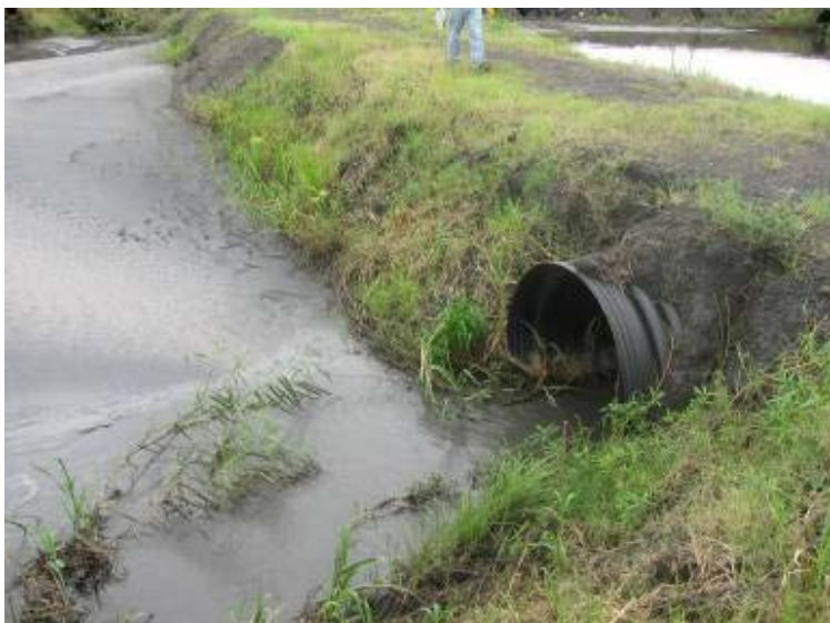
Photo 93: Interior slope, divider and equalizer pipe between Decant/Settling Ponds #3 and 4 looking northwest.
