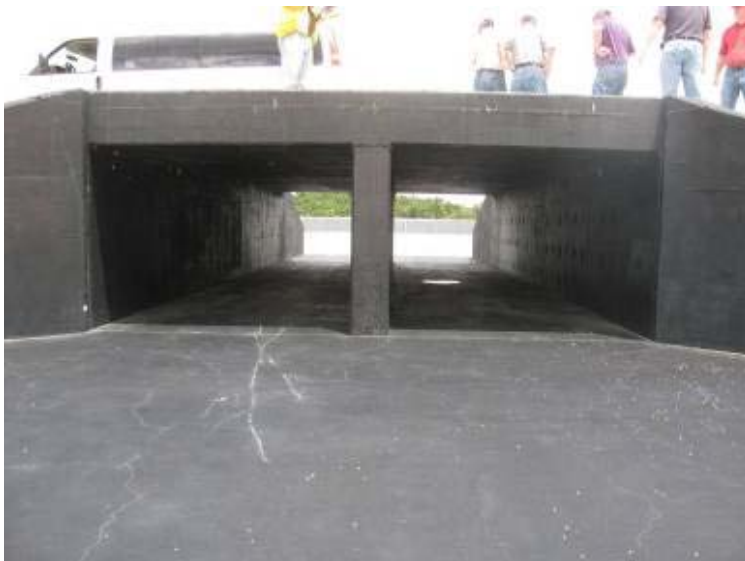
Photo 167: Concrete box culvert outlet between Gypsum Storage Pond and Process Sedimentation Pond.
