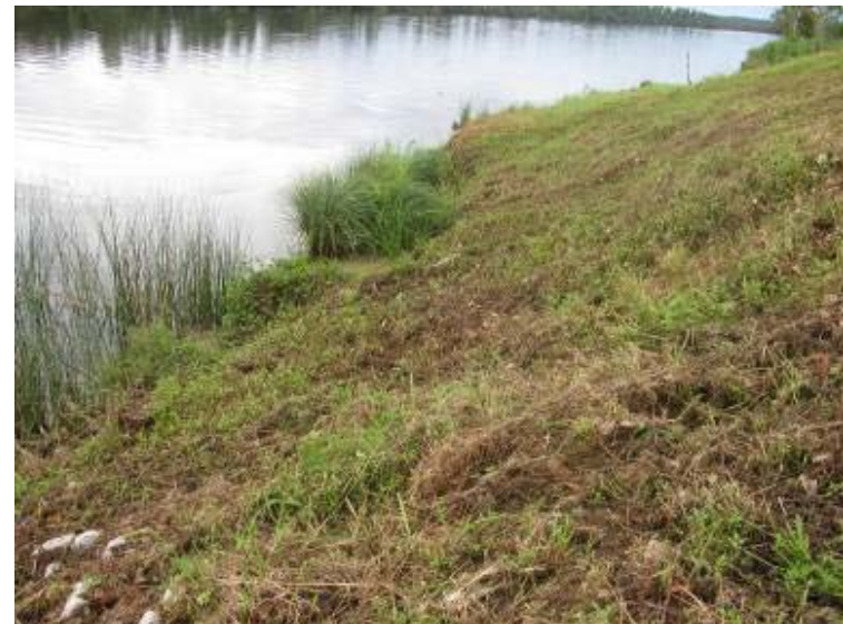
Photo 16: Erosion along toe of slope Ash Pond northeast embankment looking southeast.
