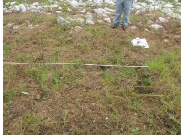
Photo 138: Three rills located along toe of north exterior slope of Process Sedimentation Pond looking north (down slope).
