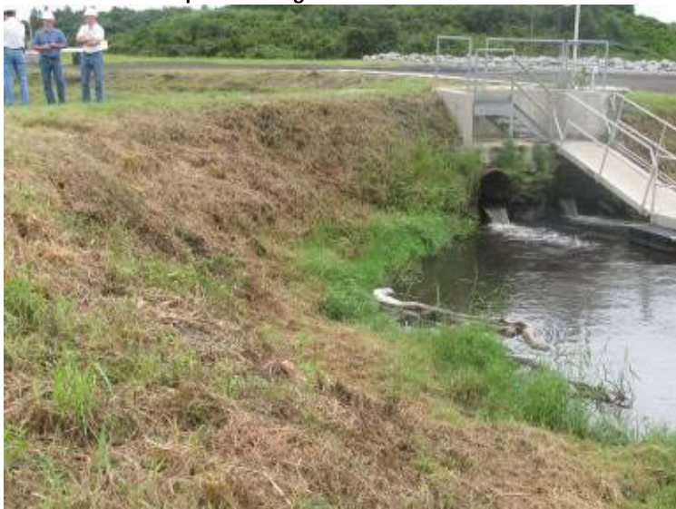
Photo 83: 30-inch diameter inlet pipes located below walkway/catwalk at north corner of Ash pond looking northwest.
