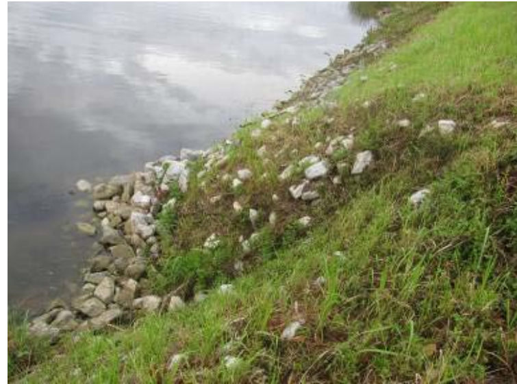
Photo 10: Erosion at toe of northeast embankment exterior slope looking southeast.
