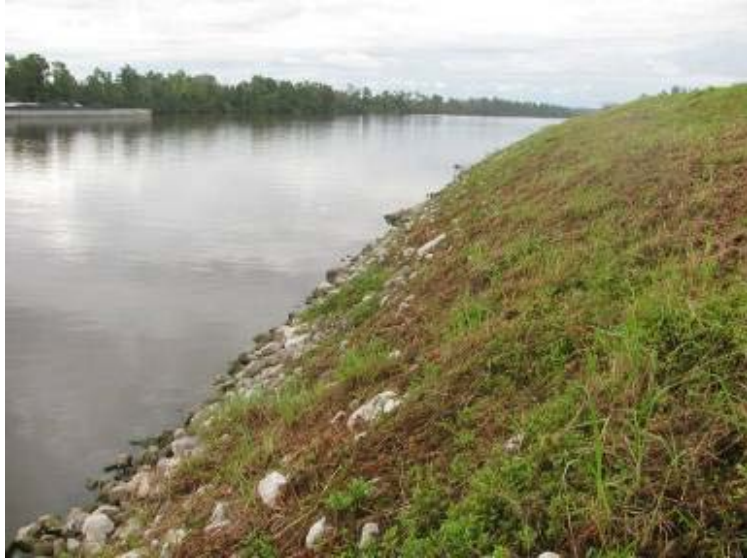
Photo 7: Ash Pond north embankment looking southeast. Note steep slope and apparent remedial works (riprap) where previous sloughing occurred.
