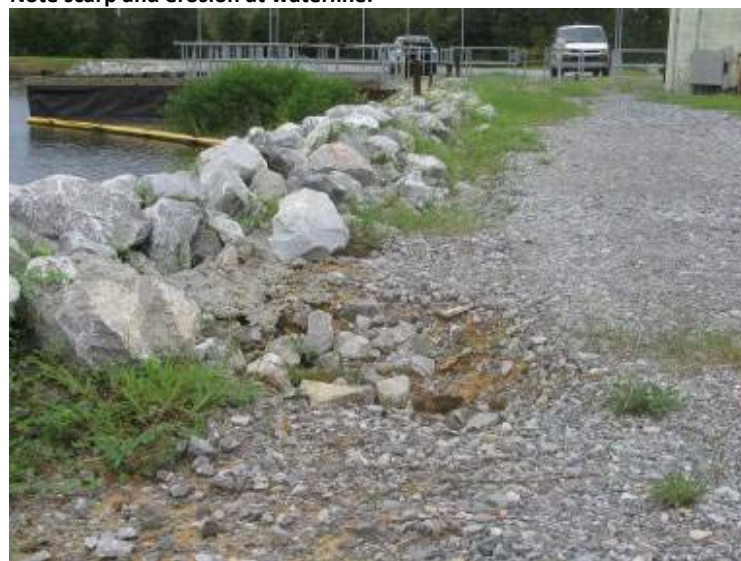
Photo 60: Settlement erosion area behind sheet pile wall and riprap on crest of Ash Pond southwest embankment. Note isolated area of loss of soil support.
