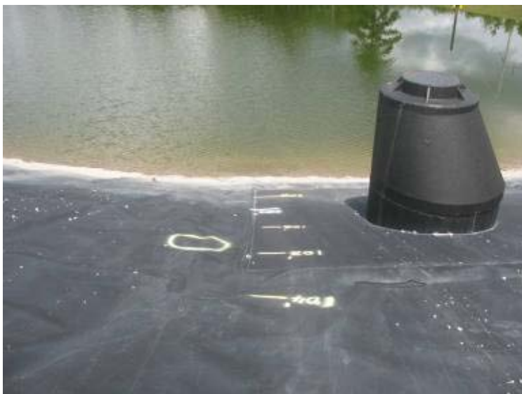
Photo 193: Manhole structure located at southwest corner of Process Return Water Pond looking east.
