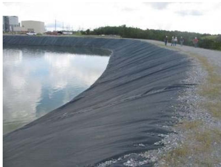
Photo 174: Textured HDPE liner on interior slope of Gypsum Storage Pond looking southeast (typical of entire pond).
