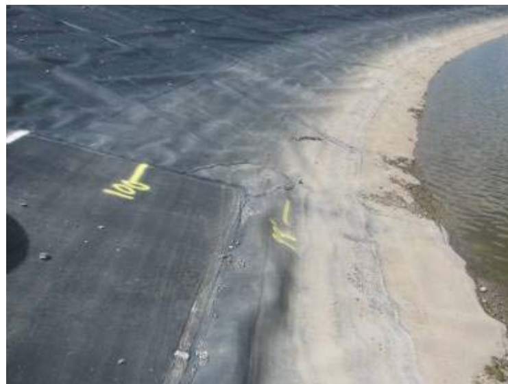
Photo 194: Textured HDPE liner on interior slope of Process Return Water Pond looking north. Note elevation data on slope.
