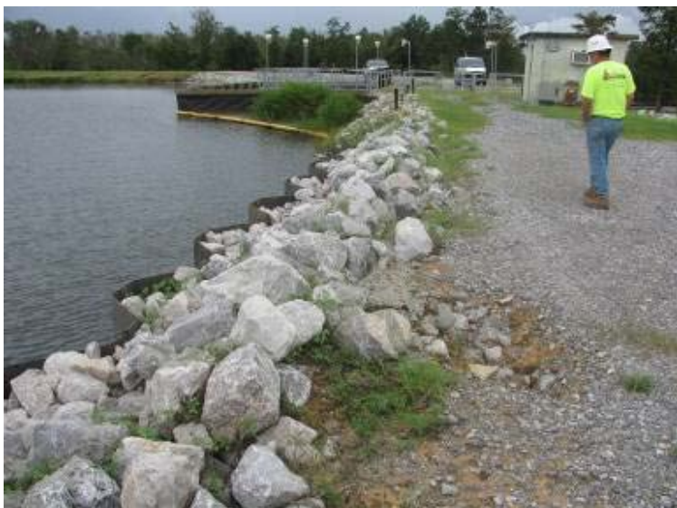
Photo 61: Erosion area behind sheet pile wall and riprap on crest of Ash Pond southwest embankment. Note isolated area of loss of soil support.
