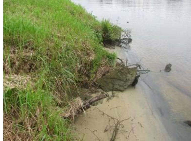
Photo 4: Close up of eroded area at exterior toe of slope adjacent to Escambia River looking northwest.
