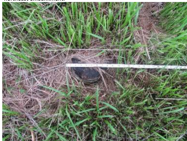
Photo 20: Tree stump found on exterior slope of Ash Pond.
