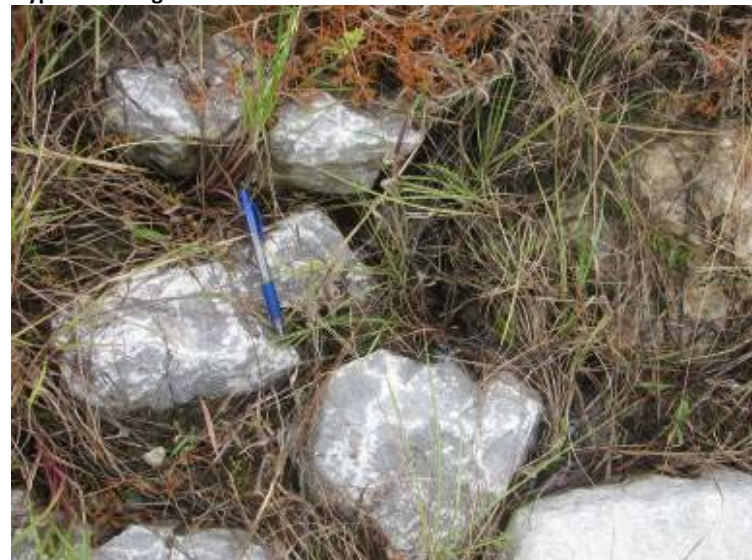
Photo 156: Wet area at toe of slope along east exterior slope of Gypsum Storage Pond.
