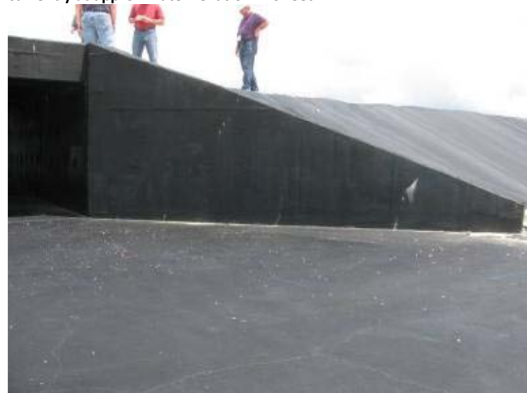
Photo 168: South wingwall of concrete box culvert outlet between Gypsum Storage Pond and Process Sedimentation Pond.
