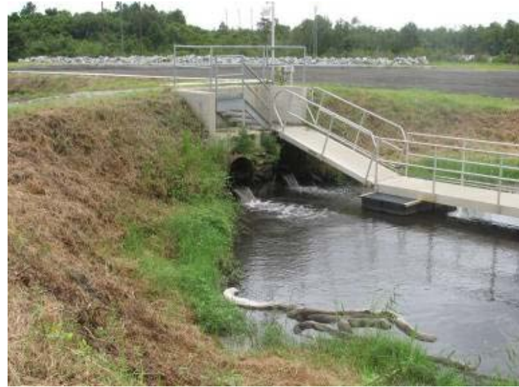
Photo 82: 30-inch diameter inlet pipes located below walkway/catwalk at north corner of Ash pond looking northwest.
