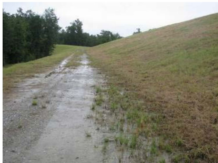
Photo 110: Perimeter road/maintenance bench at toe of SW slope of Gypsum O Pond looking northwest. Note standing water at toe.
