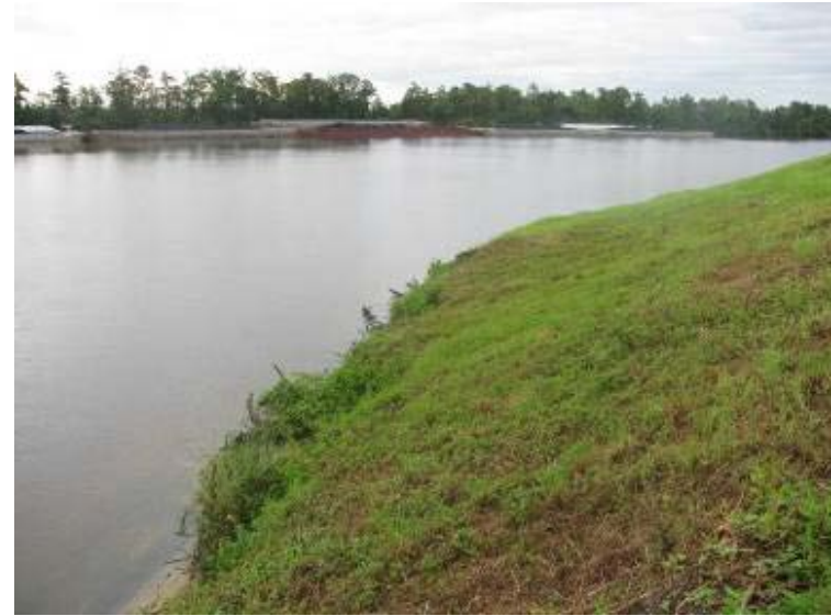
Photo 2: Ash Pond - Minor scour/erosion along toe of exterior slope of northeast embankment looking east.
