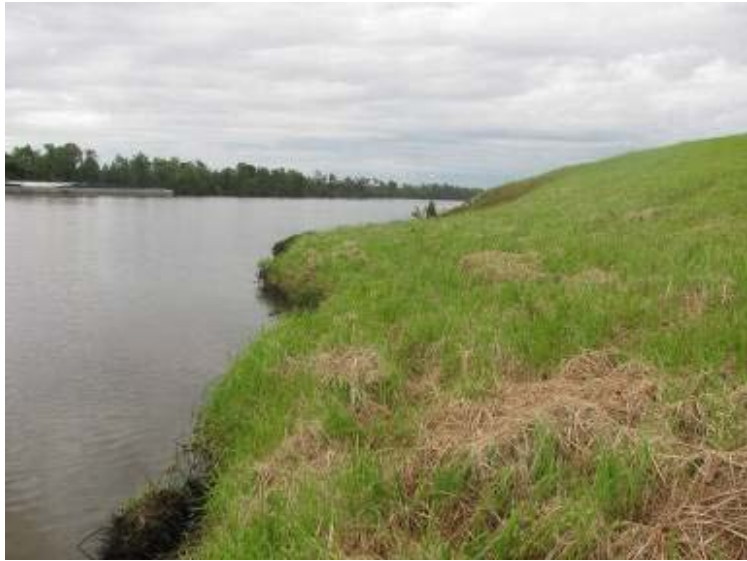
Photo 5: Scarps and erosion along the exterior slope of Ash Pond north embankment looking east.
