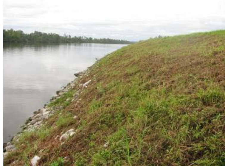
Photo 8: Ash Pond north embankment looking southeast. Note steep slope and apparent remedial works (riprap) where previous sloughing occurred.
