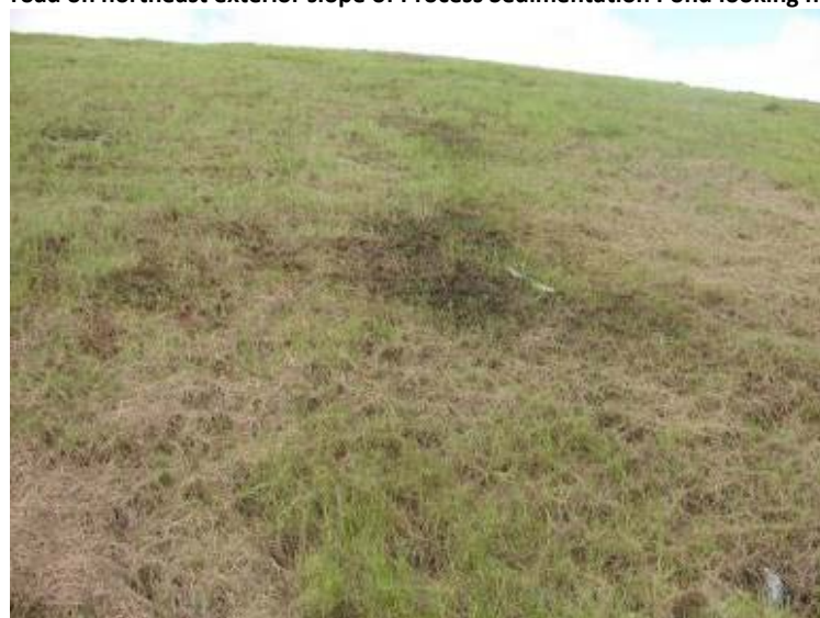
Photo 144: Wet area/possible seepage located approximately mid-slope along east exterior slope of Process Sedimentation Pond looking west.
