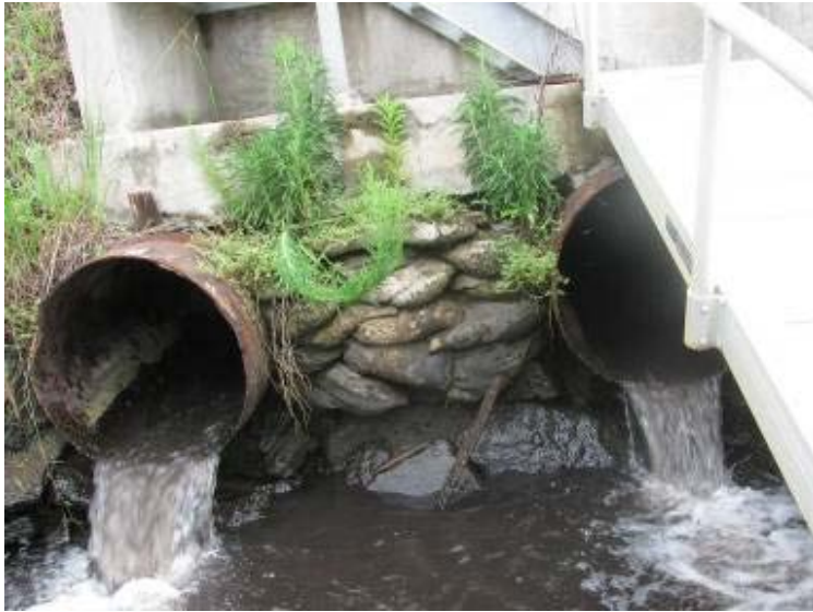
Photo 81: 30-inch diameter inlet pipes located below walkway/catwalk at north corner of Ash pond looking northwest.
