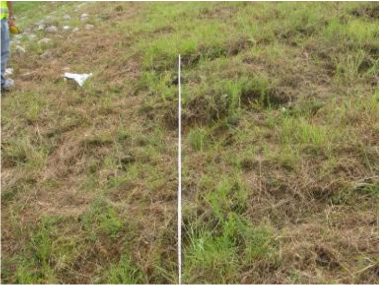
Photo 137: Three rills located along toe of north exterior slope of Process Sedimentation Pond looking east.
