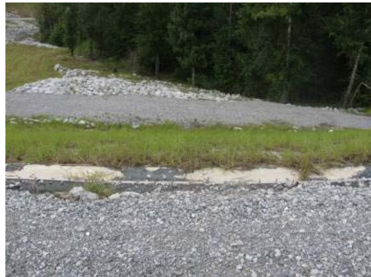
Photo 188: Emergency spillway/ACBM located on west exterior Slope of Process Return Water Pond looking west (down slope).
