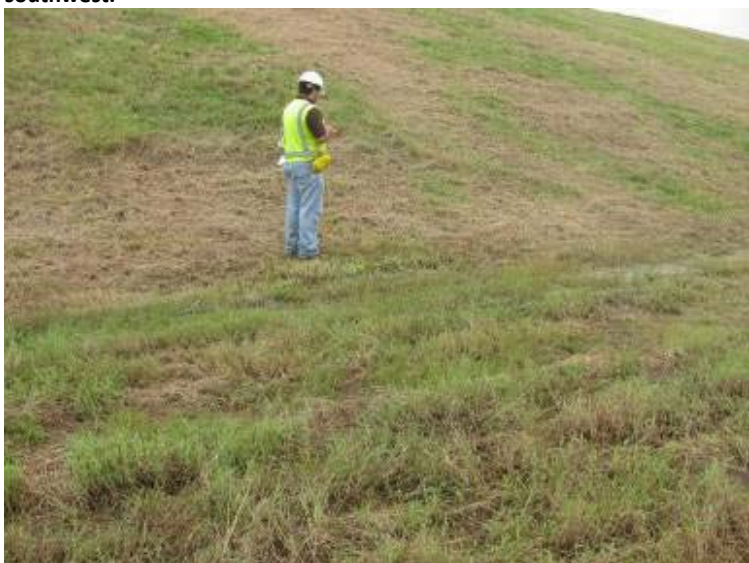
Photo 115: General view from toe of exterior slope on southwest side of Gypsum Pond looking east. Note area of wet area at toe of slope.
