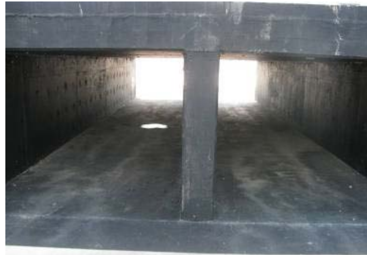
Photo 170: Concrete box culvert outlet between Gypsum Storage Pond and Process Sedimentation Pond.
