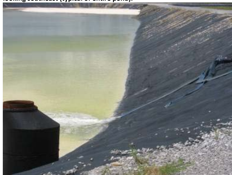
Photo 176: Inflow of water into Gypsum Storage Pond looking northwest. Note presence of textured HDPE liner on interior slope of (typical of entire pond).
