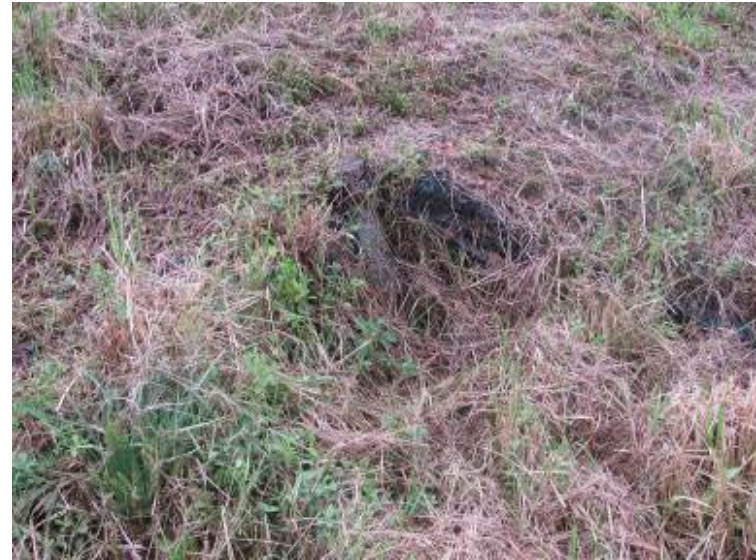
Photo 26: Southeast embankment exterior slope, tree stump and abandoned silt fence.
