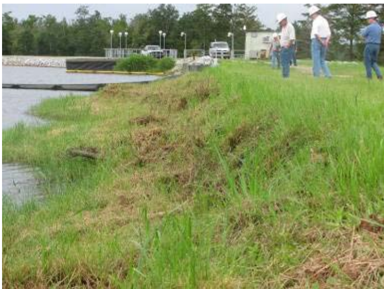
Photo 53: Interior slope scarps along Ash Pond southwest embankment looking southeast.
