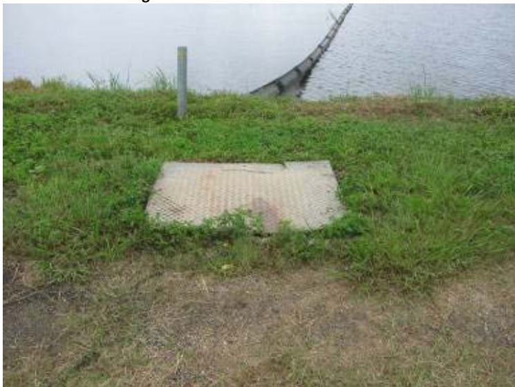
Photo 51: Electrical pull box located along Ash Pond crest of southeast embankment.
