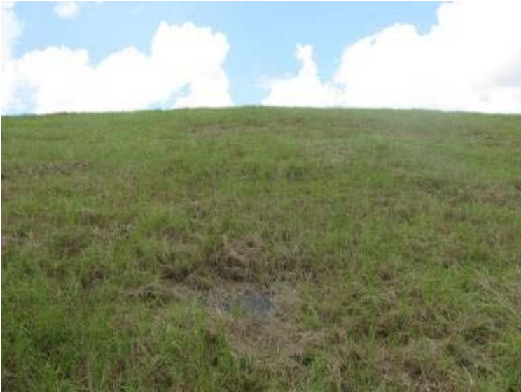
Photo 161: Scarp located on exterior slope of southeast embankment of Process Sedimentation Pond looking northwest.
