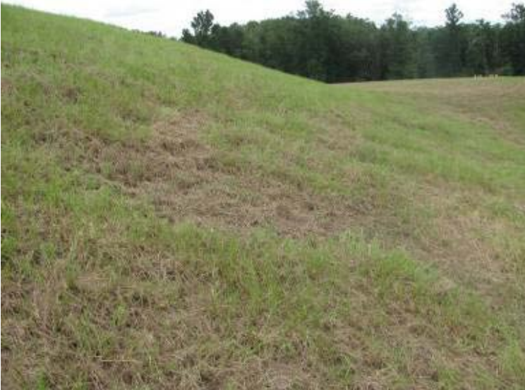
Photo 163: East exterior slope of Process Sedimentation Pond showing sloughed area looking north.
