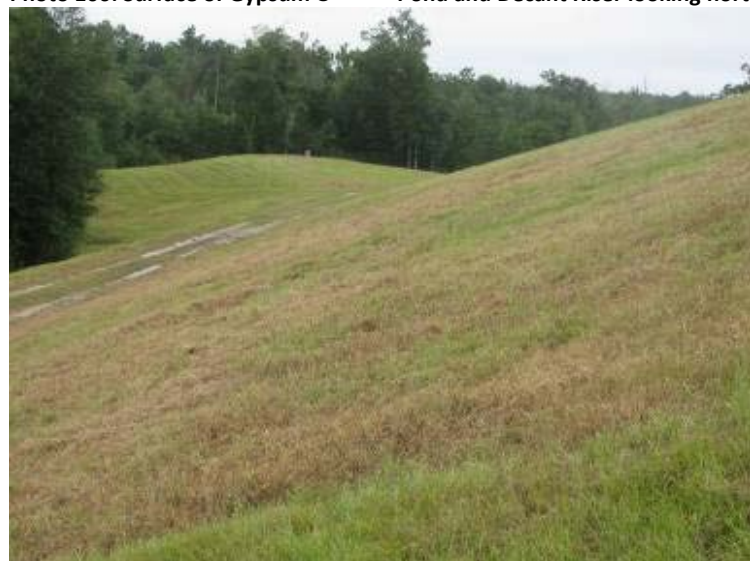
Photo 108: Exterior slope and perimeter road/maintenance bench along southwest side of Gypsum Pond looking northwest.
