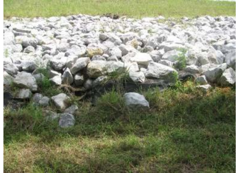
Photo 192: Riprap slope on toe of slope of northwest, exterior of Process Return Water Pond looking north. Note exposed filter fabric.
