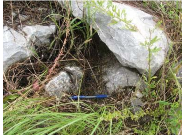
Photo 158: Wet area at toe of slope along east exterior slope of Gypsum Storage Pond.
