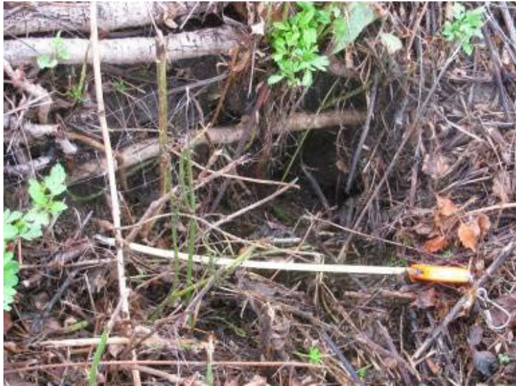
Photo 13: Animal burrow on exterior slope of Ash pond northeast embankment.
