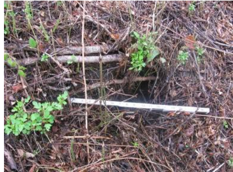
Photo 14: Animal burrow on exterior slope of Ash pond northeast embankment.
