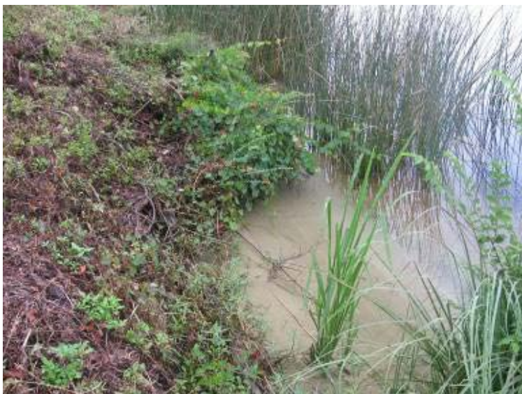
Photo 17: Scarp with sand fan at toe of slope of Ash Pond along northeast embankment.
