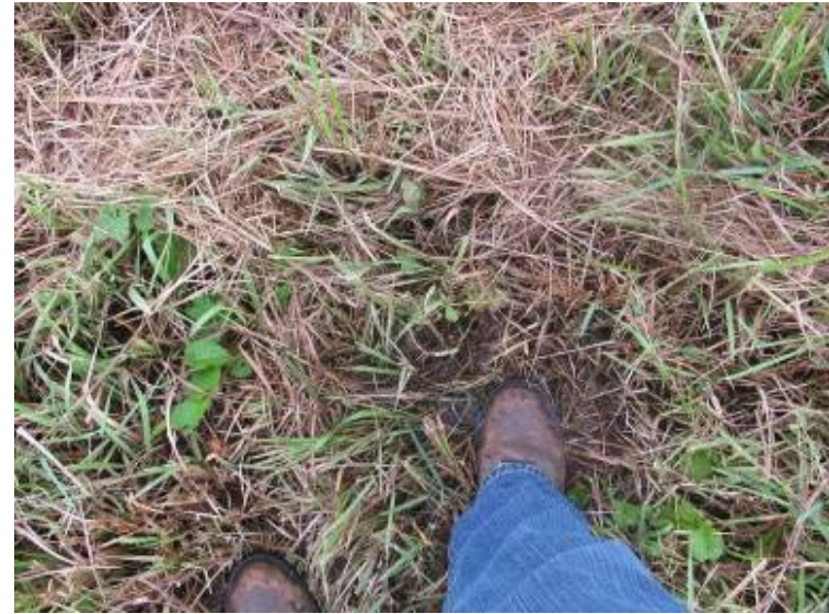
Photo 22: Area of saturation along exterior toe of slope of Ash Pond near southeast corner.
