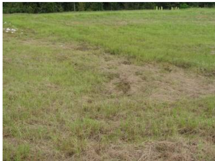
Photo 142: Wet area/saturation located at toe of slope adjacent to access road on northeast exterior slope of Process Sedimentation Pond looking north.
