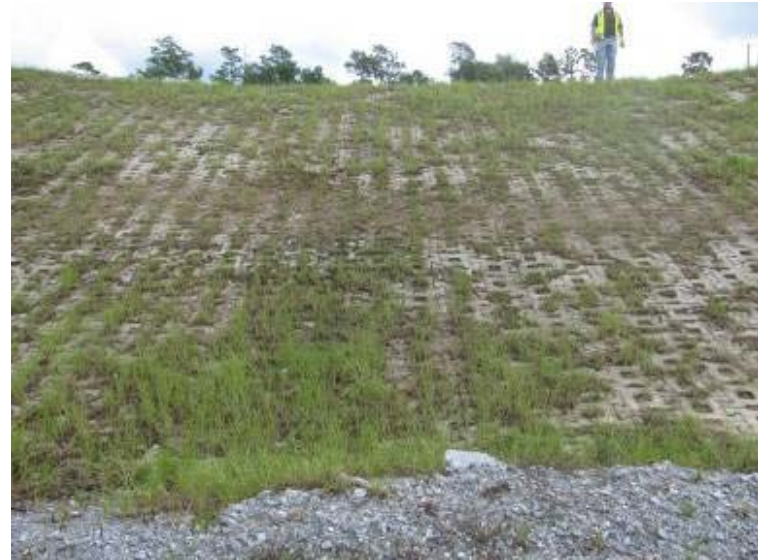
Photo 190: Emergency spillway/ACBM located on west exterior slope of Process Return Water Pond looking east (up slope).
