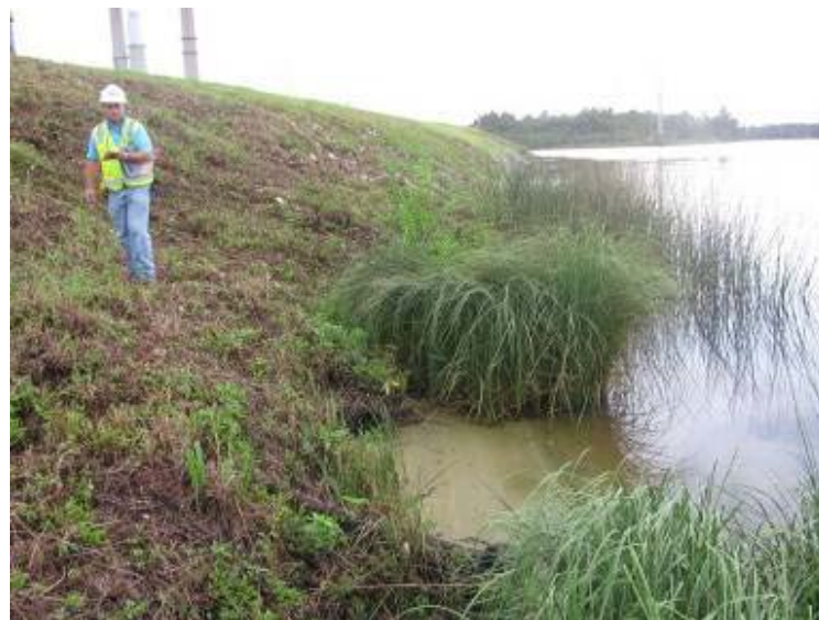
Photo 18: Scarp with sand fan at toe of slope of Ash Pond along northeast embankment.
