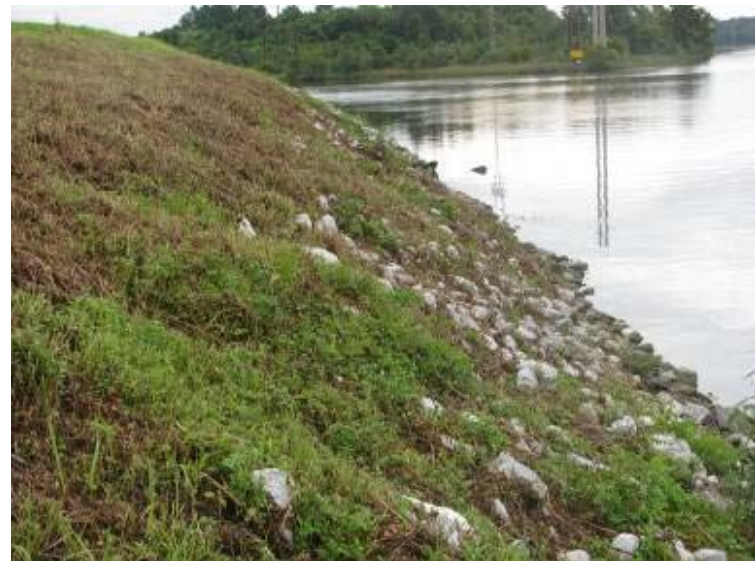
Photo 12: General view of exterior slope of Ash Pond northeast embankment looking northwest.
