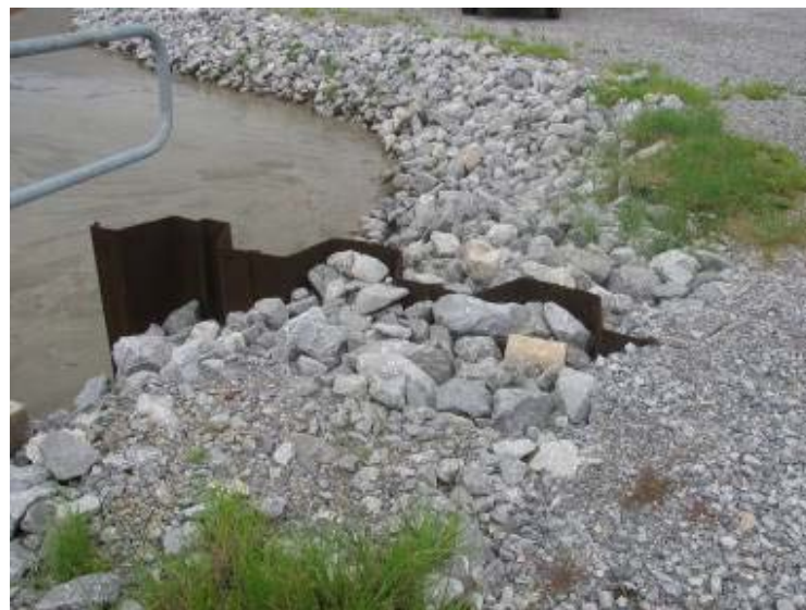
Photo 62: Portion of abandoned sheet pile cofferdam left in place on south side of spillway used to construct spillway.
