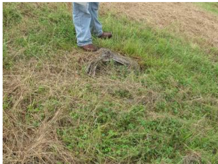
Photo 114: Trash and grass cuttings on southwest exterior slope of Gypsum Pond.
