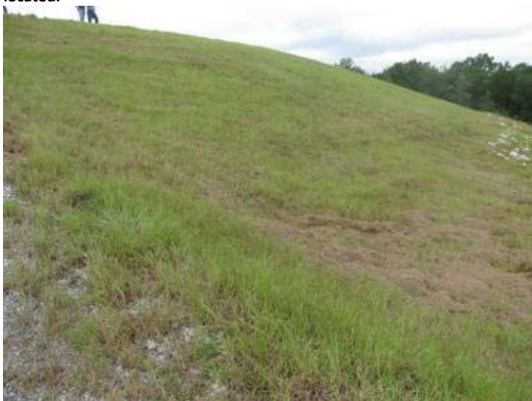
Photo 143: Wet area/saturation located at toe of slope adjacent to access road on northeast exterior slope of Process Sedimentation Pond looking east.
