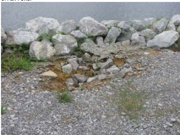
Photo 59: Settlement erosion behind sheet pile wall and riprap on crest of Ash Pond southwest embankment. Note isolated area of loss of soil support.
