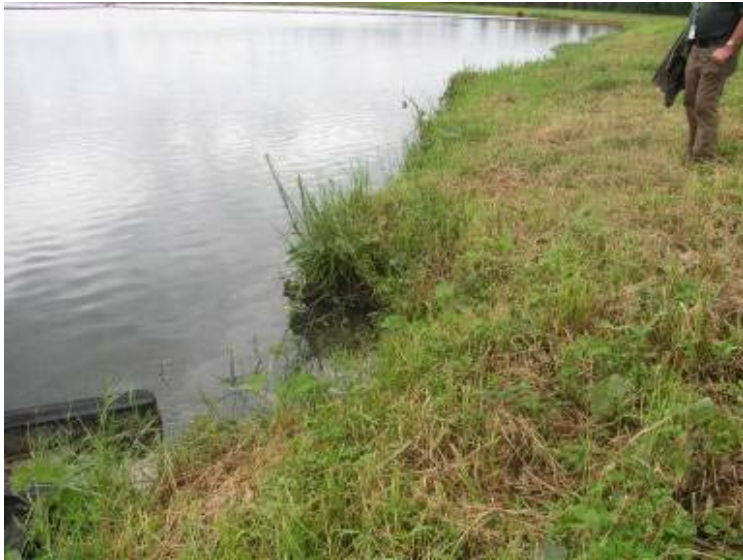
Photo 65: Erosion at interior slope and crest of Ash Pond along southeast embankment looking northeast.
