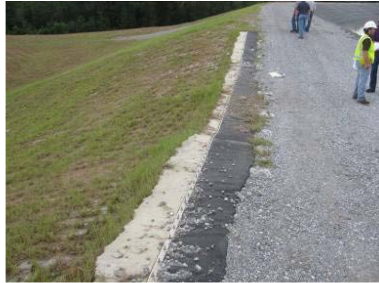
Photo 150: Top of emergency spillway along crest of east embankment of Process Sedimentation Pond.
