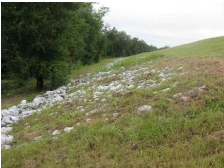
Photo 121: Start of riprap slope protection along toe of west exterior slope of Gypsum Pond looking north. Slope in this area is about 2.5H:1V.
