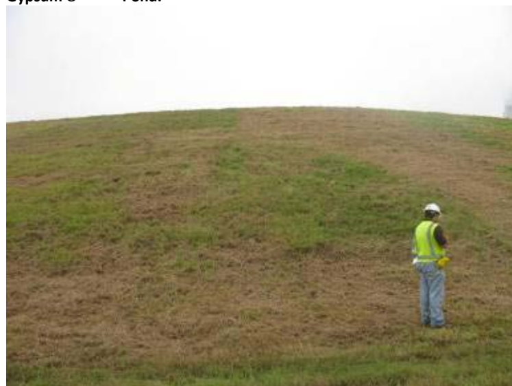
Photo 116: General view from toe of exterior slope on southwest side of Gypsum Pond looking east.
