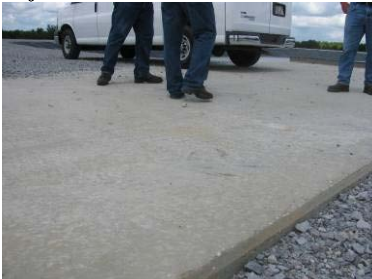
Photo 171: Concrete apron on top of concrete box culvert between Gypsum Storage Pond and Process Sedimentation Pond.
