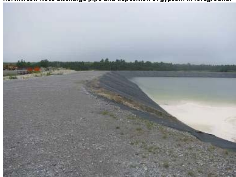
Photo 104: Crest and interior slope of south embankment of Gypsum Pond looking southwest.
