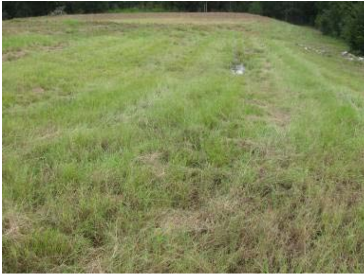
Photo 145: Area of wet area/possible seepage located approximately mid-slope along east exterior slope of Process Sedimentation Pond looking east.
