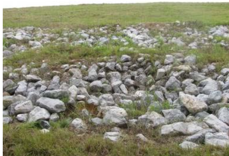
Photo 122: Riprap slope protection along toe of west exterior slope of Gypsum Pond looking east. Note depressed area at center.
