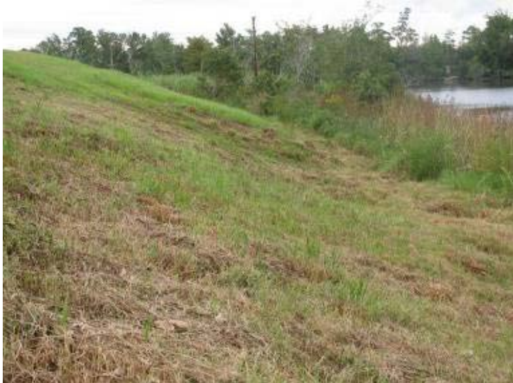
Photo 27: Exterior slope of Ash Pond along southeast embankment looking southwest. Note depression due to erosion.
