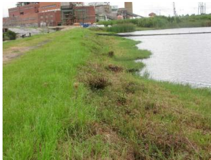
Photo 58: Southwest embankment interior slope looking northwest. Note scarp and erosion at waterline.
