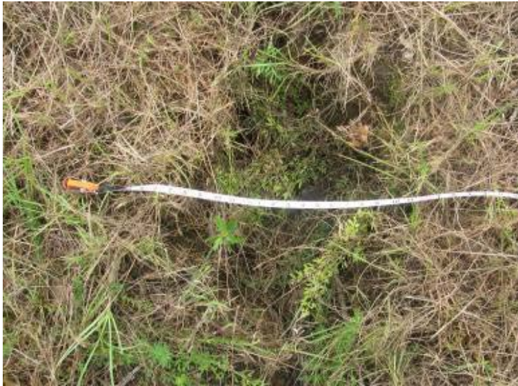
Photo 133: Approximate 16-foot long rill erosion on north exterior Slope of Process Sedimentation Pond (width is about 1 foot).
