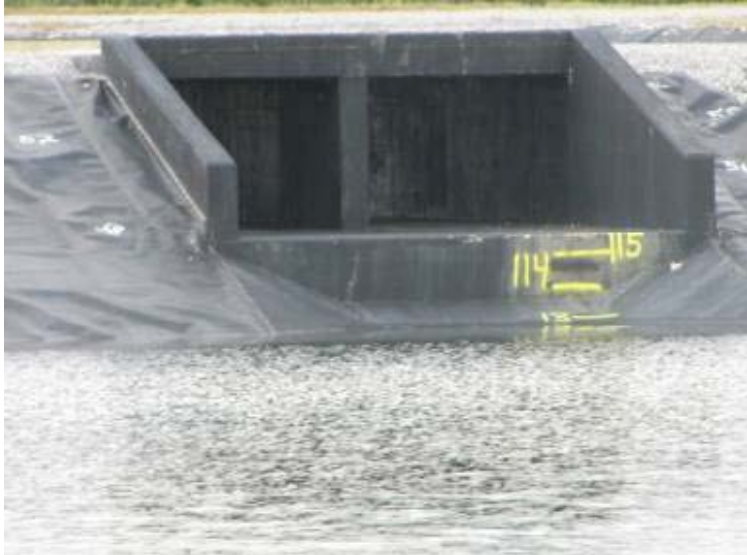
Photo 151: Concrete box culvert discharge between Gypsum Storage Pond and Process Sedimentation Pond.
