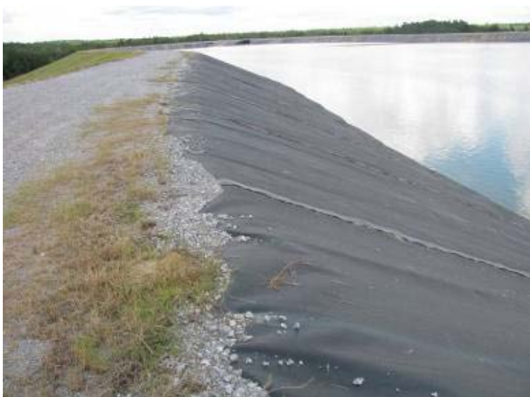
Photo 175: Textured HDPE liner on interior slope of Gypsum Storage Pond looking northwest (typical of entire pond).
