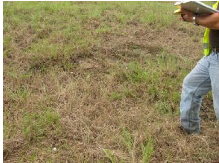
Photo 162: Wet area/potential seepage located on exterior slope near southeast corner Process Sedimentation Pond.
