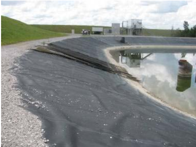
Photo 181: South crest and interior slope of Process Return Water Pond looking west.
