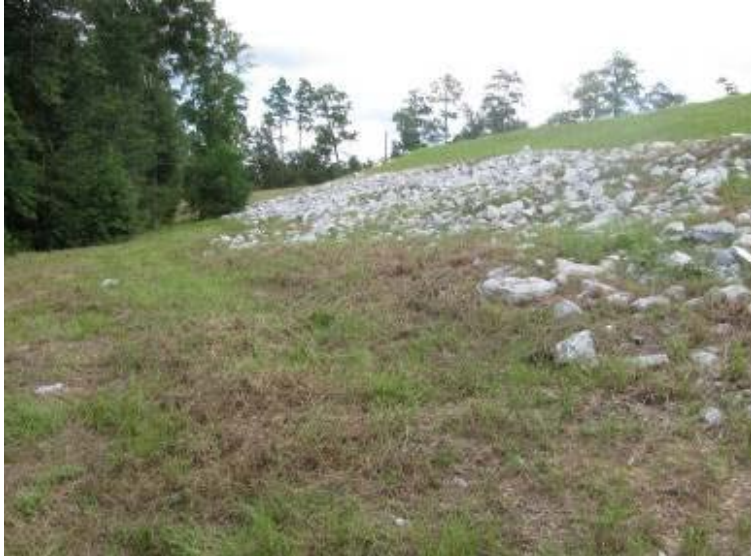
Photo 191: Riprap slope treatment along toe of slope of northwest, exterior of Process Return Water Pond looking north.
