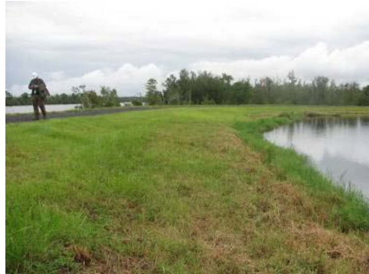
Photo 70: Interior slope and crest of Ash Pond along northeast embankment looking south.
