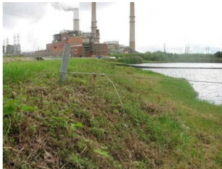
Photo 54: Interior slope scarps along Ash Pond southwest embankment looking northwest. Note steepness and discontinuity of eroded slope.
