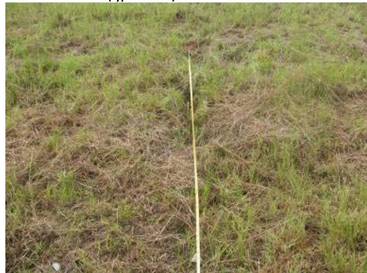
Photo 136: Rill located near toe of north exterior slope of Process Sedimentation Pond looking southeast (up slope).
