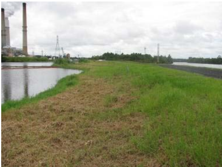
Photo 71: Interior slope and crest of Ash Pond along northeast embankment looking northwest.
