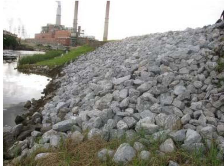
Photo 46: Exterior toe of slope of Ash Pond along southwest embankment looking northwest.
