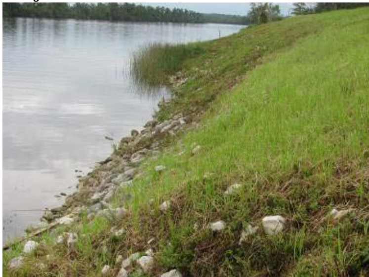
Photo 11: General view of exterior slope of Ash Pond northeast embankment looking southeast.
