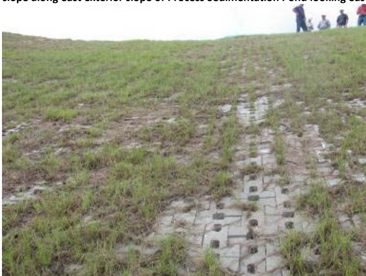
Photo 147: Emergency spillway/articulated concrete block mattress located on east ext.slope of Process Sed. Pond looking west (up slope).
