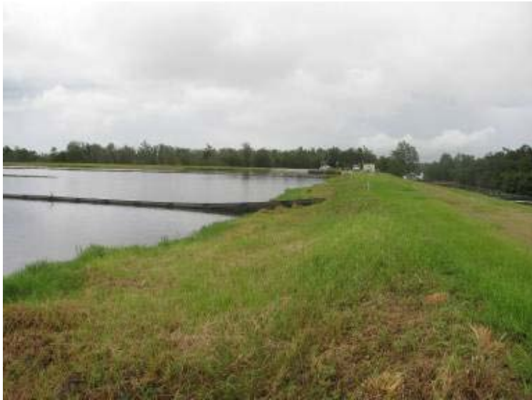
Photo 49: Interior slope and crest of Ash Pond along southwest embankment looking southeast.
