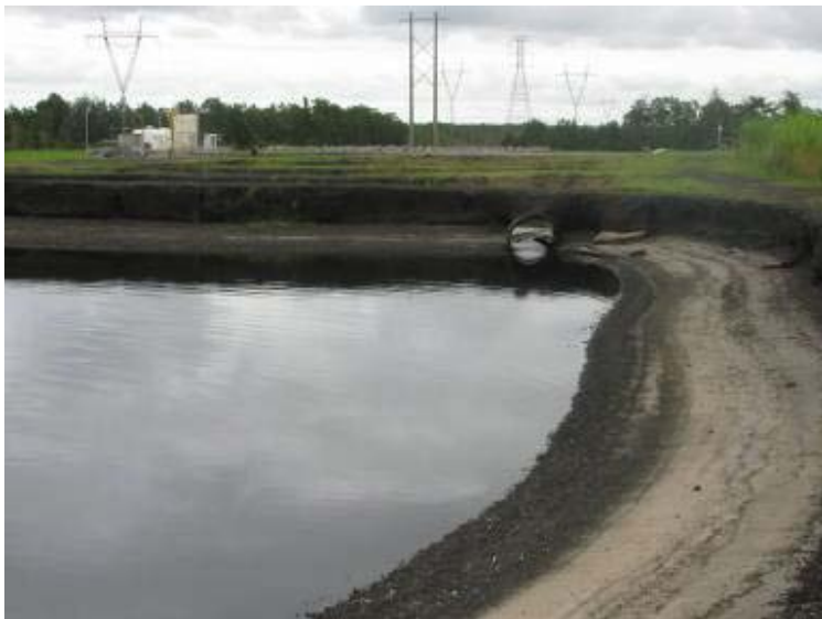
Photo 87: Interior slopes and surface of Decant/Settling Pond #1 looking northeast. Note equalizer pipe between ponds.
