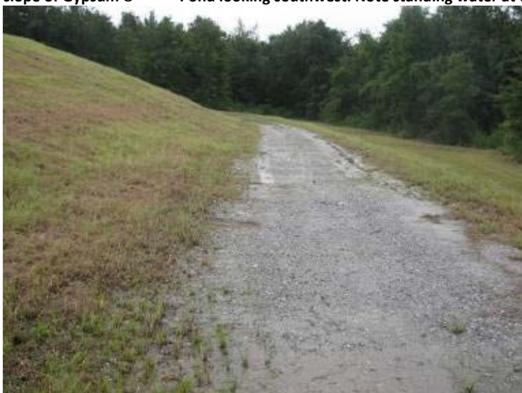
Photo 111: Perimeter road/maintenance bench at toe of southwest slope of Gypsum O Pond looking southwest. Note standing water at toe.
