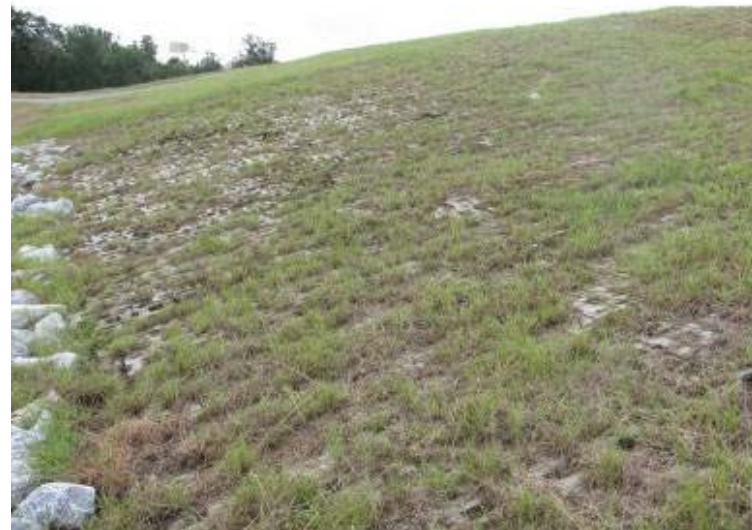
Photo 148: Emergency spillway/articulated concrete block mattress located on east ext. slope of Process Sed. Pond looking south.
