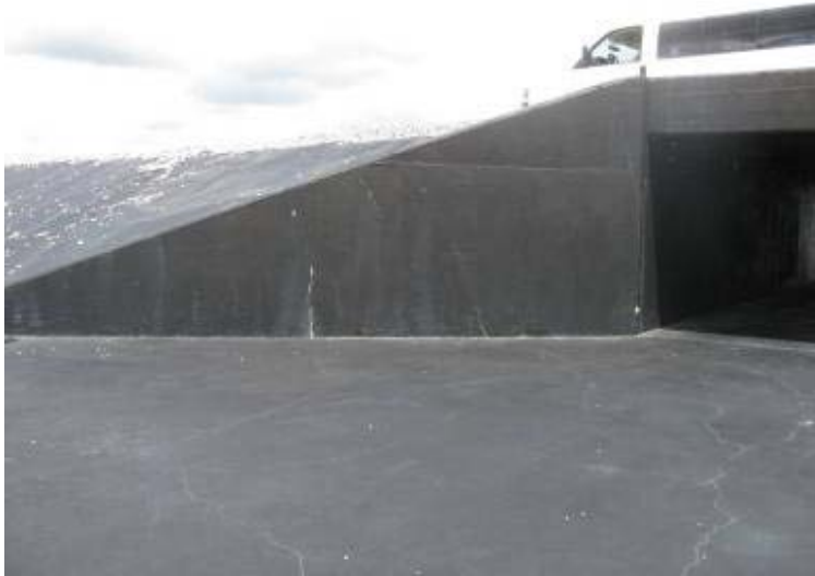
Photo 169: North wingwall concrete box culvert outlet between Gypsum Storage Pond and Process Sedimentation Pond.
