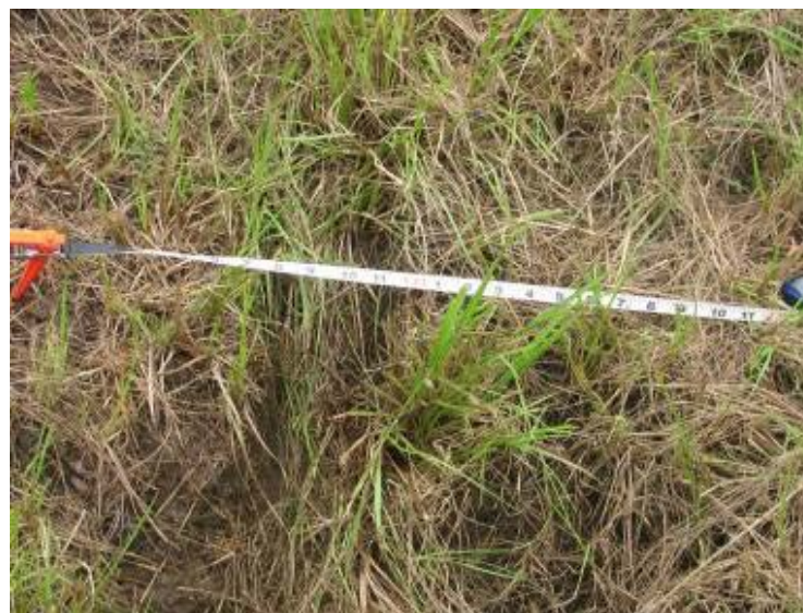
Photo 128: Rill located at approximate mid-face of west exterior slope of Gypsum O Pond. Depth is about 4 to 6 inches.
