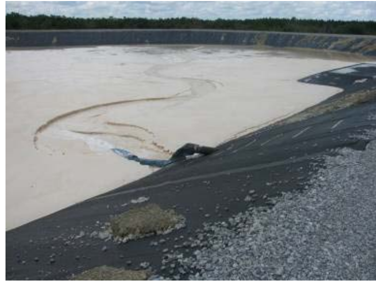
Photo 166: Discharge pipe into Gypsum Storage Pond. Gypsum and water currently at approximate Elevation 113 feet.
