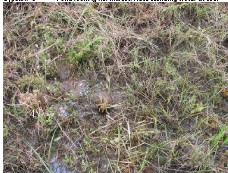
Photo 112: Close-up of wet area/possible seepage at toe of southwest Slope of Gypsum O Pond.
