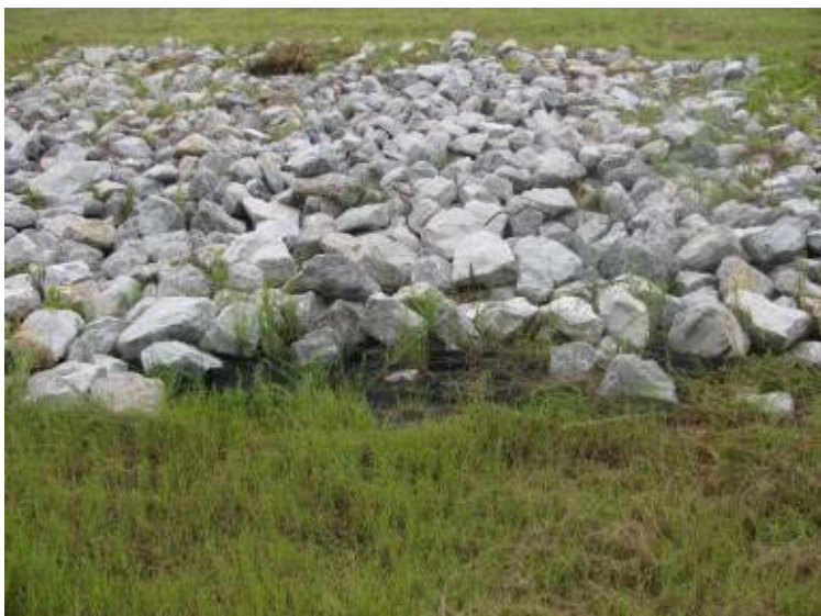
Photo 141: Exposed filter fabric beneath riprap where a depression is located.
